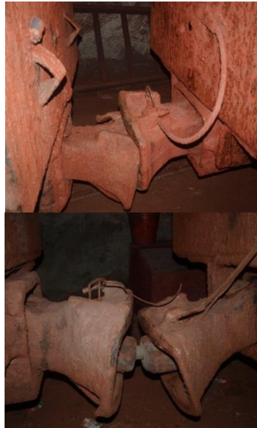
Fig. 1. Photographic evidence of conditions of drawbars of VG-4.5 cars (for two extreme positions)
